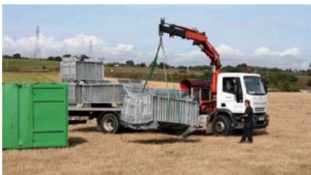
Day 2 The fencing arrives and later in the day the chemical toilets make their appearance.
